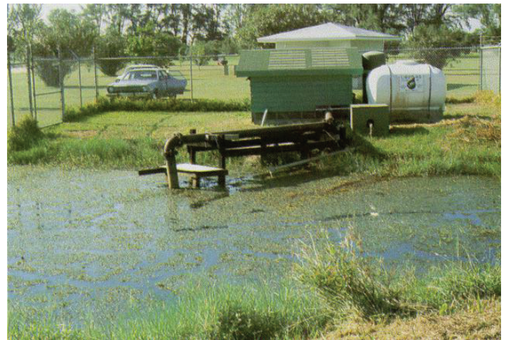
Figure 1. Dense Hydrilla growth can seriously impact agricultural operations, shown here blocking the intake line of an irrigation pump. Credits: David L. Sutton
